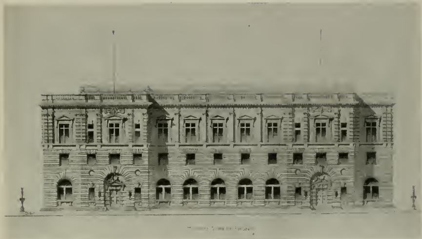
SAN FRANCISCO POST-OFFICE, IN COURSE OF CONSTRUCTION, CORNER SEVENTH AND MISSION STREETS.
